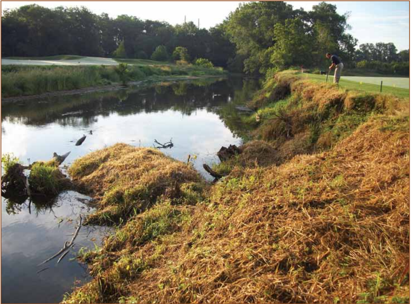
Stream bank at the start of the project, demonstrating severe high bank erosion, undercutting and slumping as well as invasive vegetation.
