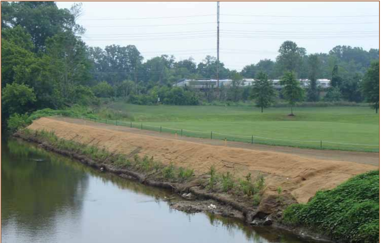
The final piece of the design was to maintain a stable toe of bank using a combination of coir fiber logs, low growing shrubs and a heavy jute mat (same area as photo on page 8).
